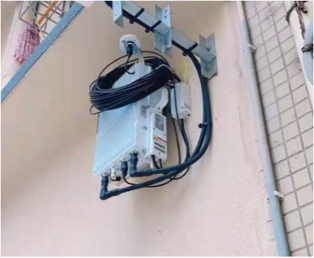
GPS antenna blocked
