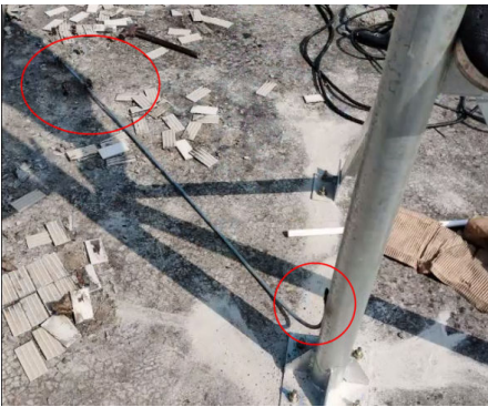
The holding pole lightning rod is not led to the ground bar
