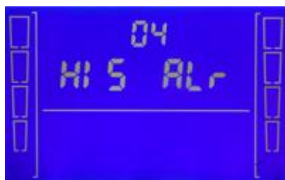
Figure 4-9 Historical alarm display menu
