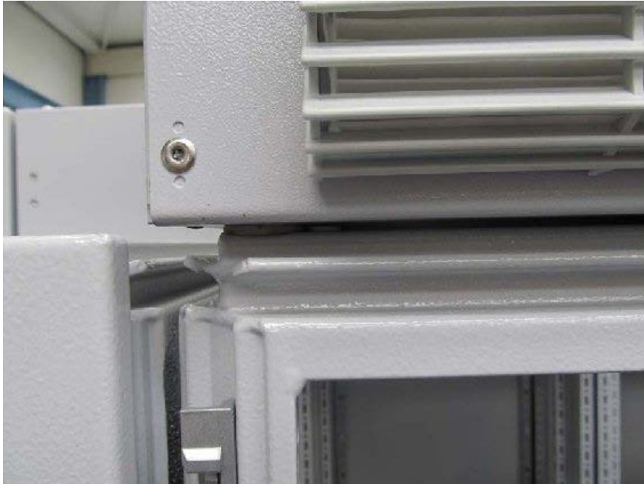
Figure 3-19 View with opened cabinet door
