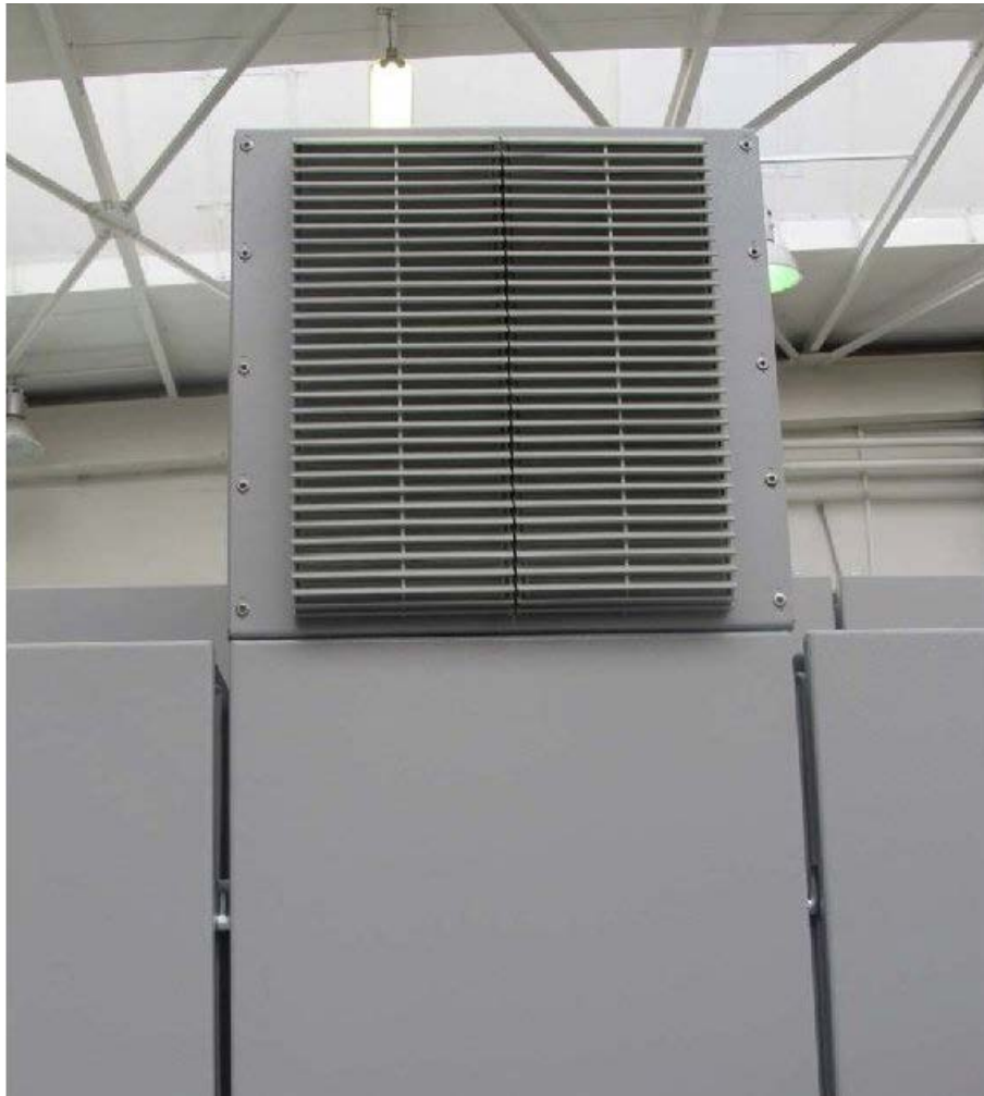
Figure 3-20 View with closed cabinet door
