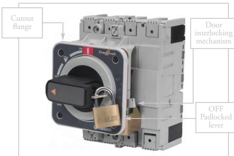
Breaker Mounted Handle Padlocked in the OFF Position
