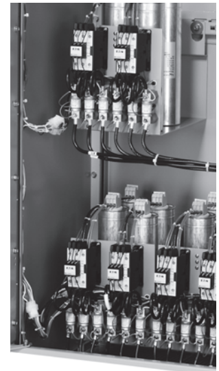
Factory Pre-Wired for Future Expansion
