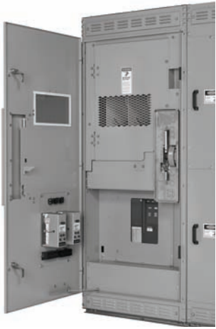
Indoor Medium Voltage Switch and Fixed Breaker—MSB
