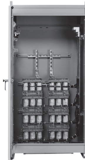
AUTOVAR Filter—Reactor Cabinet
