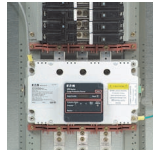
Surge Protective Devices can be Integrated within a variety of Eaton Electrical Assemblies
