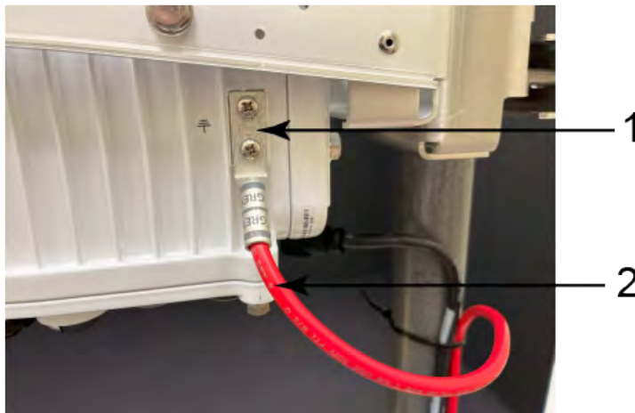
Figure 36 6AWG ground cable and ground lug location
