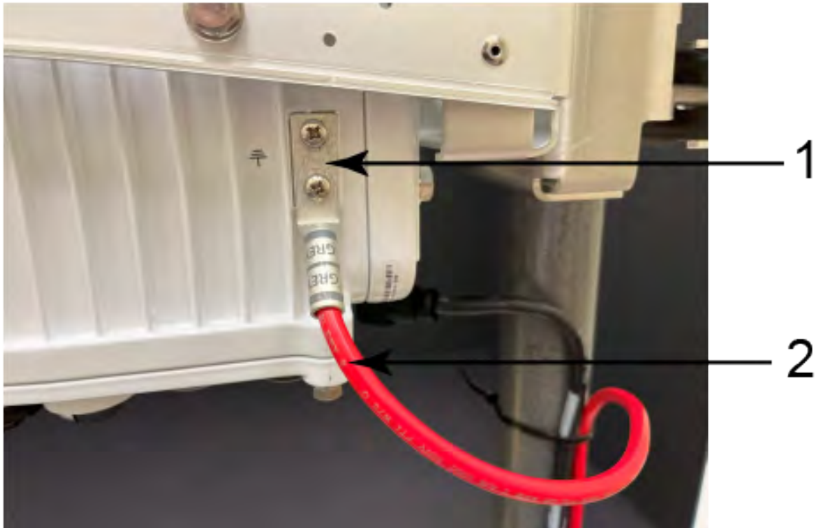
Figure 10 6AWG Ground cable and ground lug location
