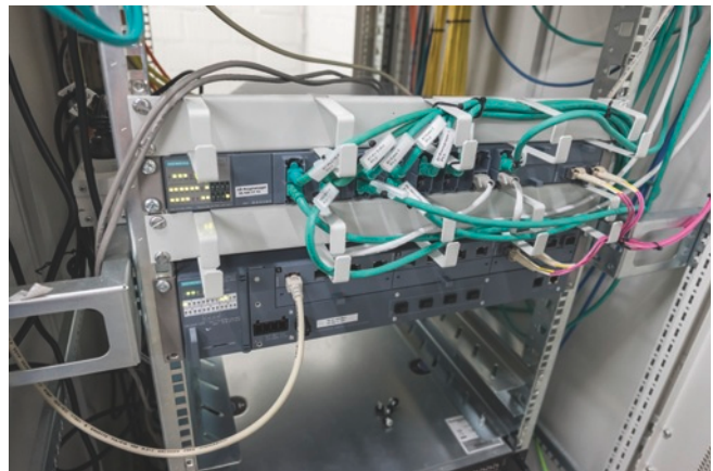
The SCALANCE X switches are installed in decentralized control cabinets.
