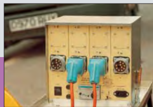
Telephone line connections
