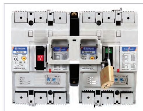
Slide Interlock Installed Between two MCCBs
