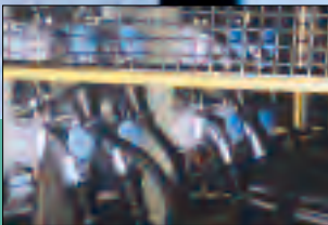
Power supply to production lines
