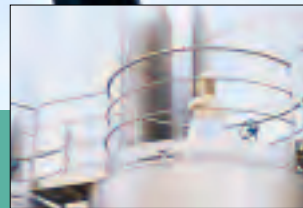
Power supply to motors and pumps
