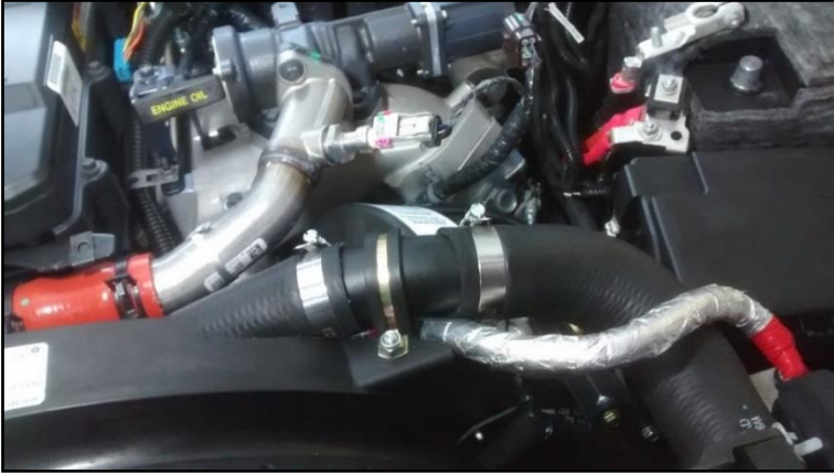
Figure 26 - Connecting the upper radiator hose
