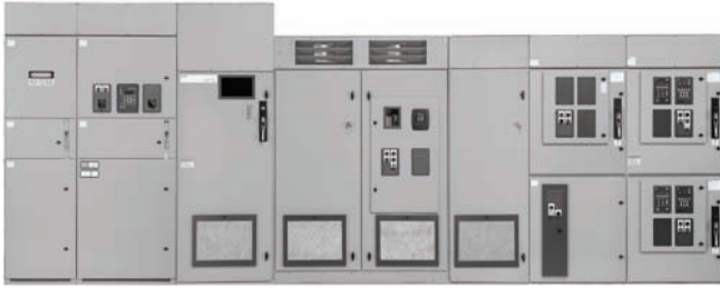
AMPGARD Motor Control Assembly with Main Breaker, SC 9000 AFD, RVSS and Two-High FVNR
