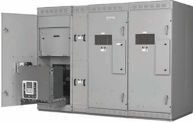
Indoor Metal-Enclosed Drawout Vacuum Breaker—MEB Used as Main for Two Fused Switches
