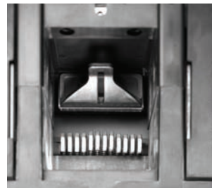
Magnum DS Breaker Contacts (Arc Chutes Removed)
