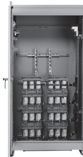
AUTOVAR Filter—Reactor Cabinet
