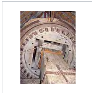
Windshaft, brake wheel, and brake blocks in smock mill d'Admiraal in Amsterdam
