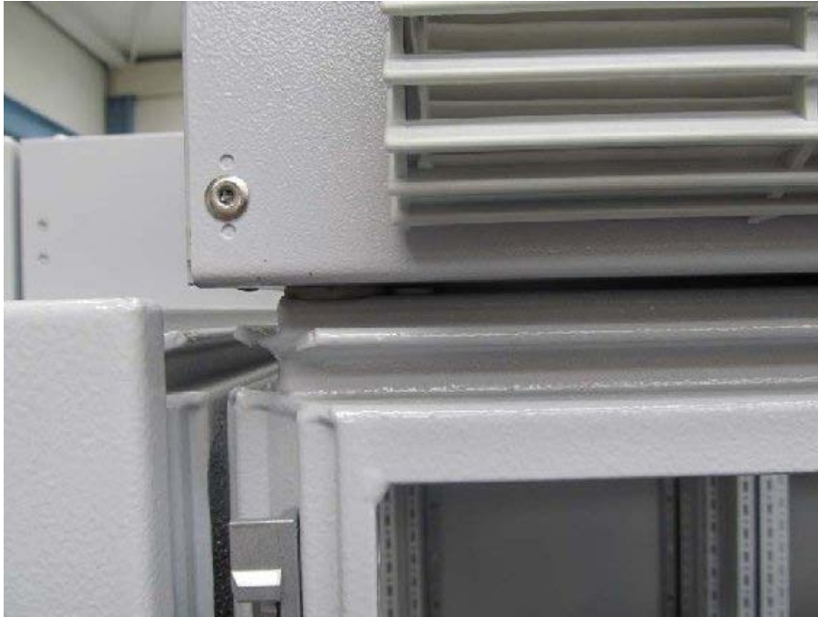
Figure 3-19 View with opened cabinet door
