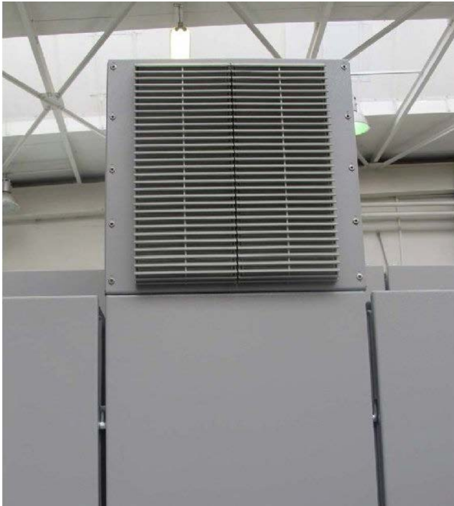
Figure 3-20 View with closed cabinet door
