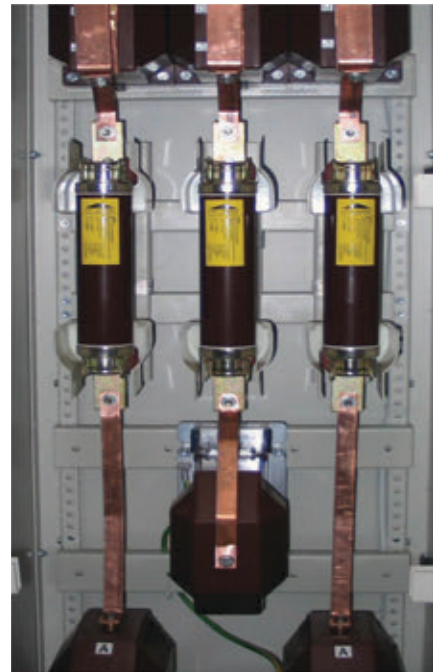
Connection in indoor switchgear, example:
